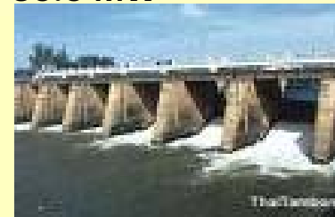
Mae Klong Dam 12.0 MW
